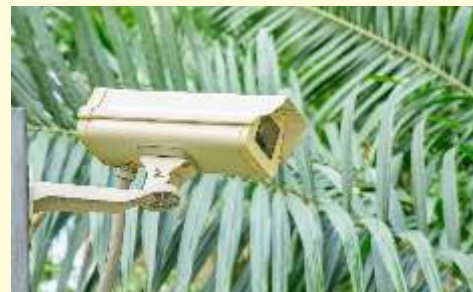
24 hrs. Security with CCTV
